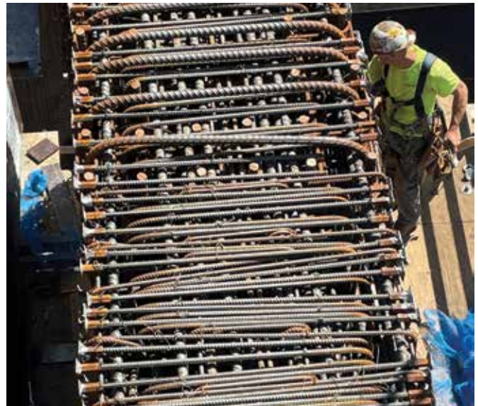
Fig. 8: Reinforcing bar density for this member was close to 800 lb/yd 3 . After this was built, the engineer changed bar sizes, bundled bars, and rearranged splices so there was access for concrete placement
