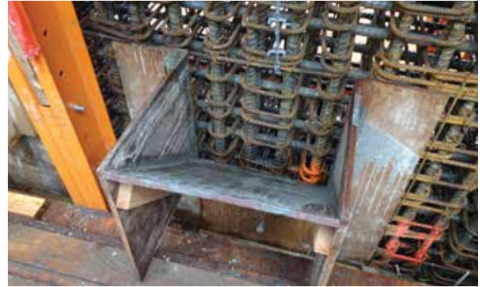
Fig. 5: Portable concrete placement chute, 16 in. wide by 12 in. deep, used at the top of the wall to allow SCC to be placed through the side of congested shear wall. Several jobsite-built wood chutes were leapfrogged to keep in front of the placing crew. Preconstruction mockup cores taken through reinforcing steel at the bottom of congested boundary elements indicated no aggregate separation
