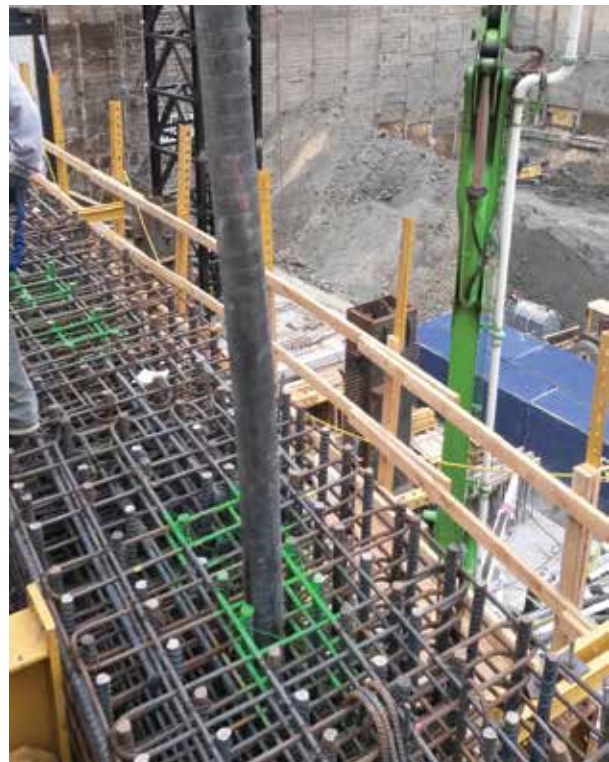
Fig. 3: Pump hose and vibrator access zones (green paint) at the top of a congested shear wall. These zones were spaced 10 ft apart over the top of the wall and were continuous over the full height of the wall. The zones were coordinated in advance with the engineer and inspection agency
