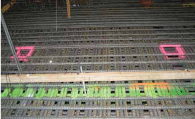
Fig. 4: Concrete pump hose access zones (pink paint). These zones were 6 in. square and were spaced 8 to 10 ft apart. Typically, top bars in both layers were shifted into proper design position and secured after pumping of the lower mat was complete. Temporary shifting of top layer reinforcing was coordinated in advance with the engineer and inspection agency
