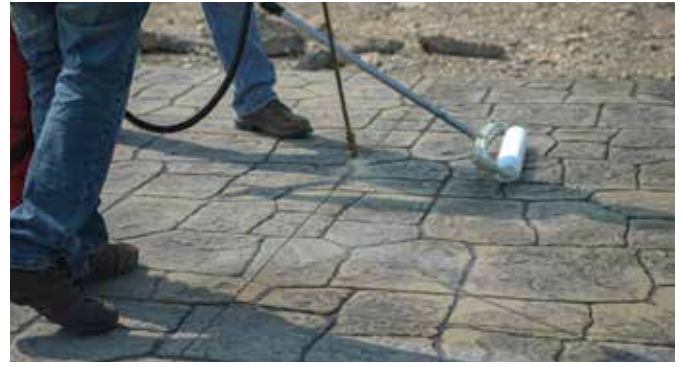
A “spray and back roll” application of a sealer on a stamped concrete surface
